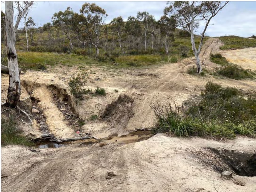
Figure 16-1: Erosion at Farmers Creek
