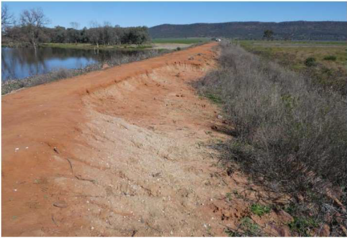
Levee K has been heavily eroded
