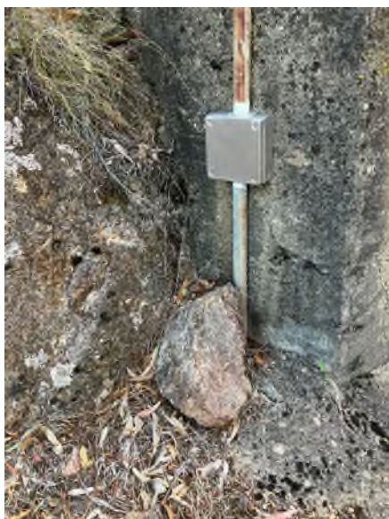
Figure 4: Junction Box for supply cables
