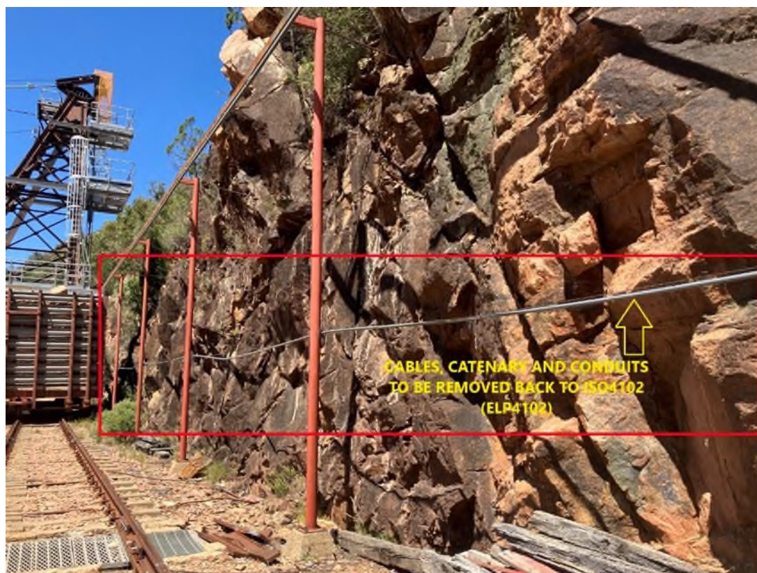
Figure 38: Redundant equipment to be removed.
