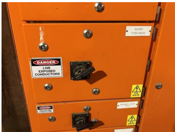
Figure 11: Feeder Circuit Isolator
