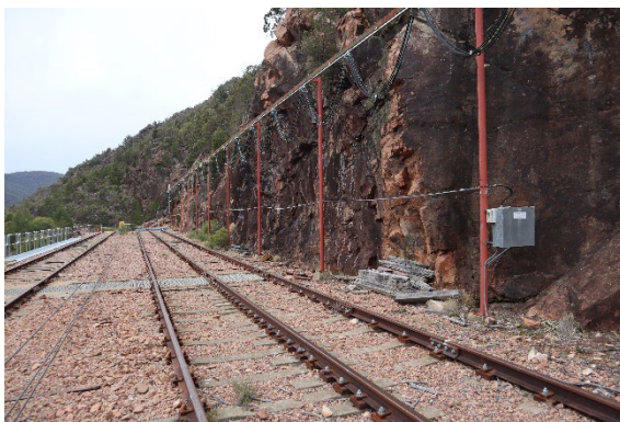
Figure 4.13 Festoon cable and mount, southern tower. On right is tower distribution board DB2. (Source: WaterNSW, July 2025)
