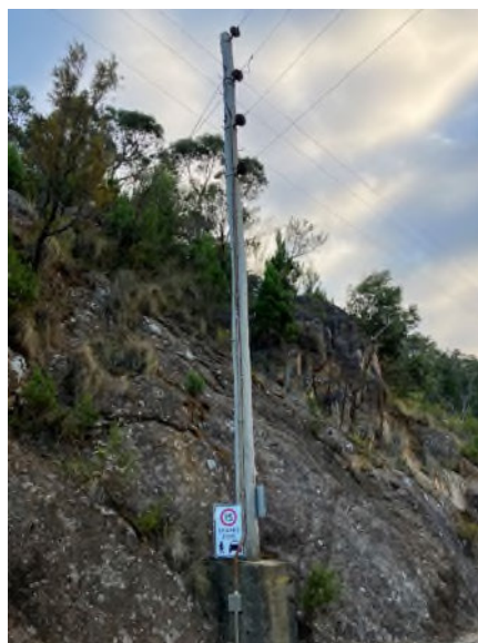
Figure 5: Pole and Aerial Conductors
