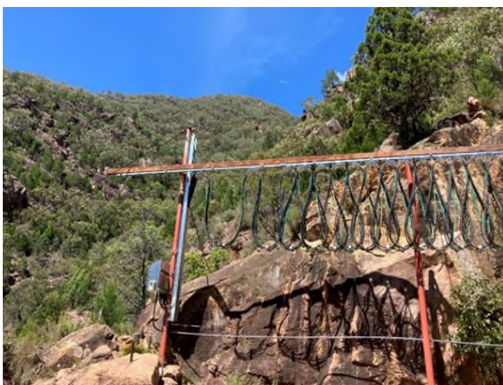
Figure 35: Festoon Cable at maximum compression (Tower has reached end stop limits)
