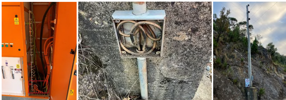
Figures 44-45: Redundant supply to be removed from SB1 to top of Northern Wooden Pole
