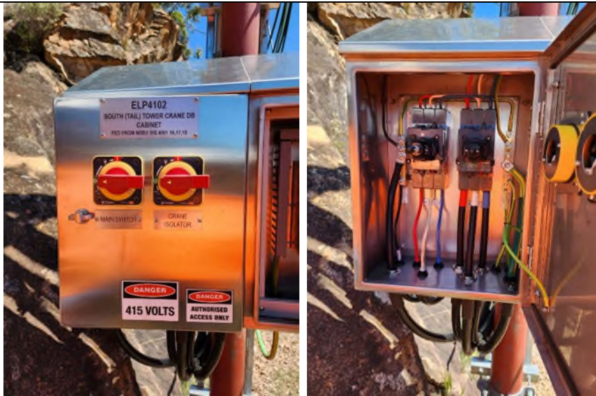
Figures 30 and 31: Main Switch and Crane Isolator
