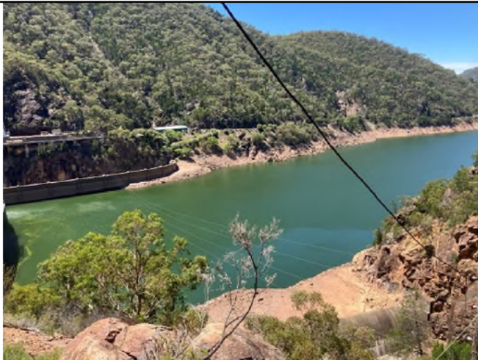
Figure 6: Aerial Conductors, Pole and Overhead Cable to Isolator
