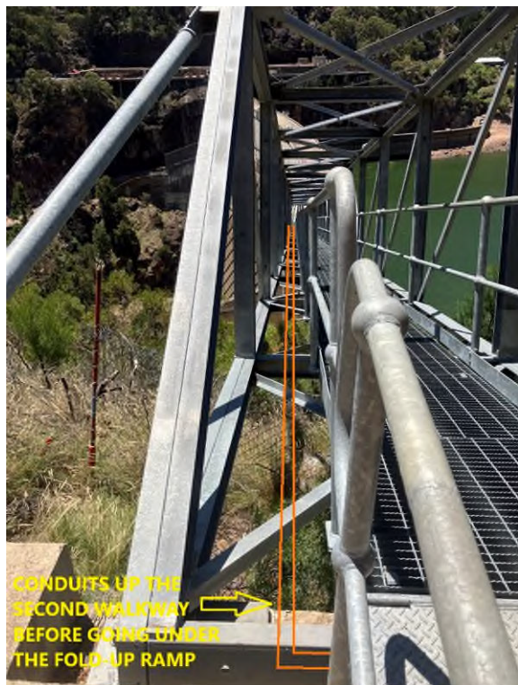
Figure 22: Conduits up 2 nd walkway
