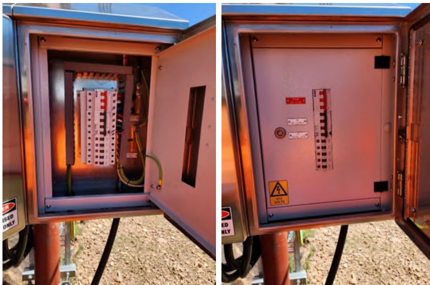
Figures 32 and 33: Breakers for Distribution Board Halfway along and Local Single Phase Outlet on Side
