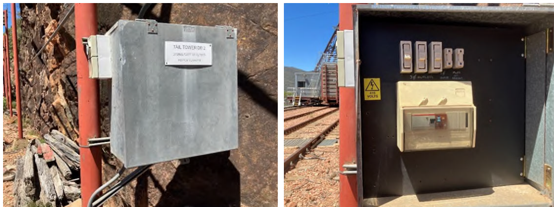
Figures 36 and 37: Tail Tower Distribution Board DB2 – to be removed
