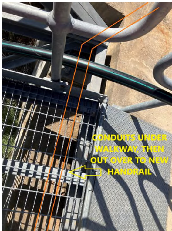
Figure 23: Conduits going under walkway
