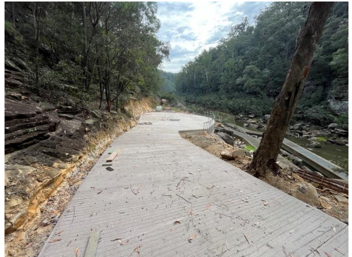
Repairs to the access track at Theresa Park Weir near the fishway.
