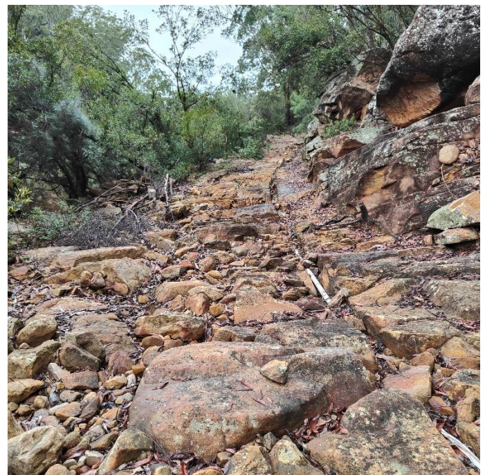
The access track prior to repairs. This section will be stabilised and upgraded with a concrete surface.
