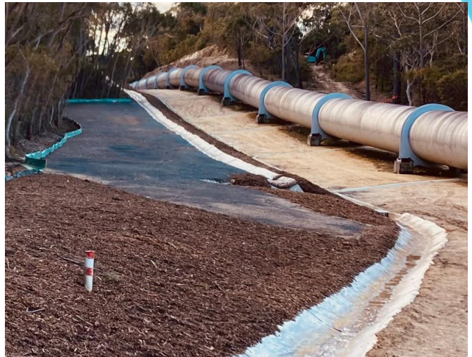
Stage one works on the Kangaroo Valley pipeline included bearing replacement and drainage works
