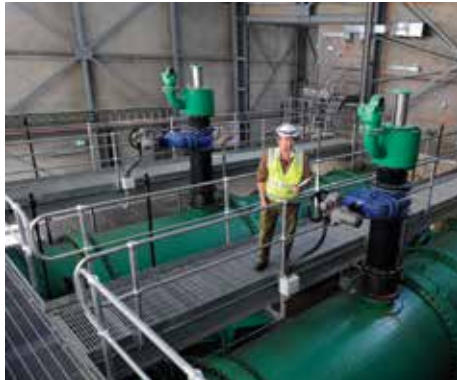
^ THE VALVE HOUSE, WARRAGAMBA
