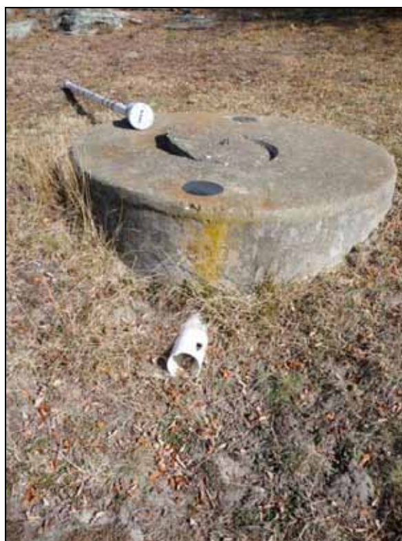
Figure 3.8 Outlet pipe discharging directly onto open ground
