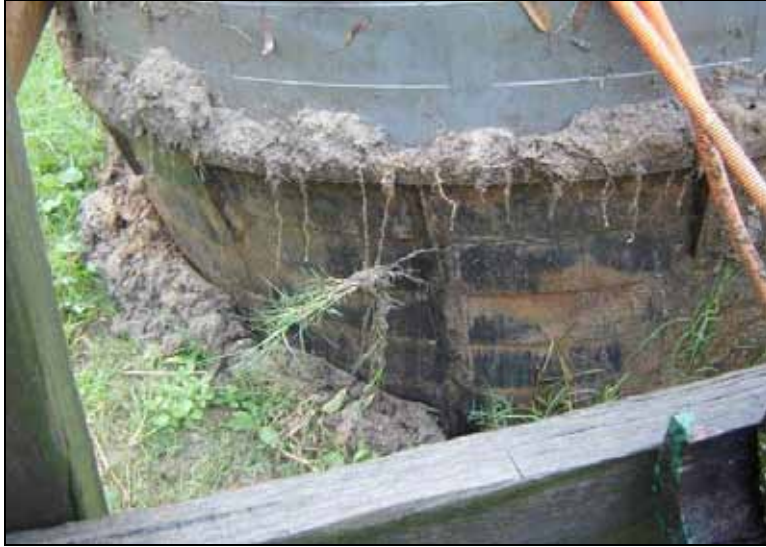
Figure 3.9 Tank that has lifted due to high water table
