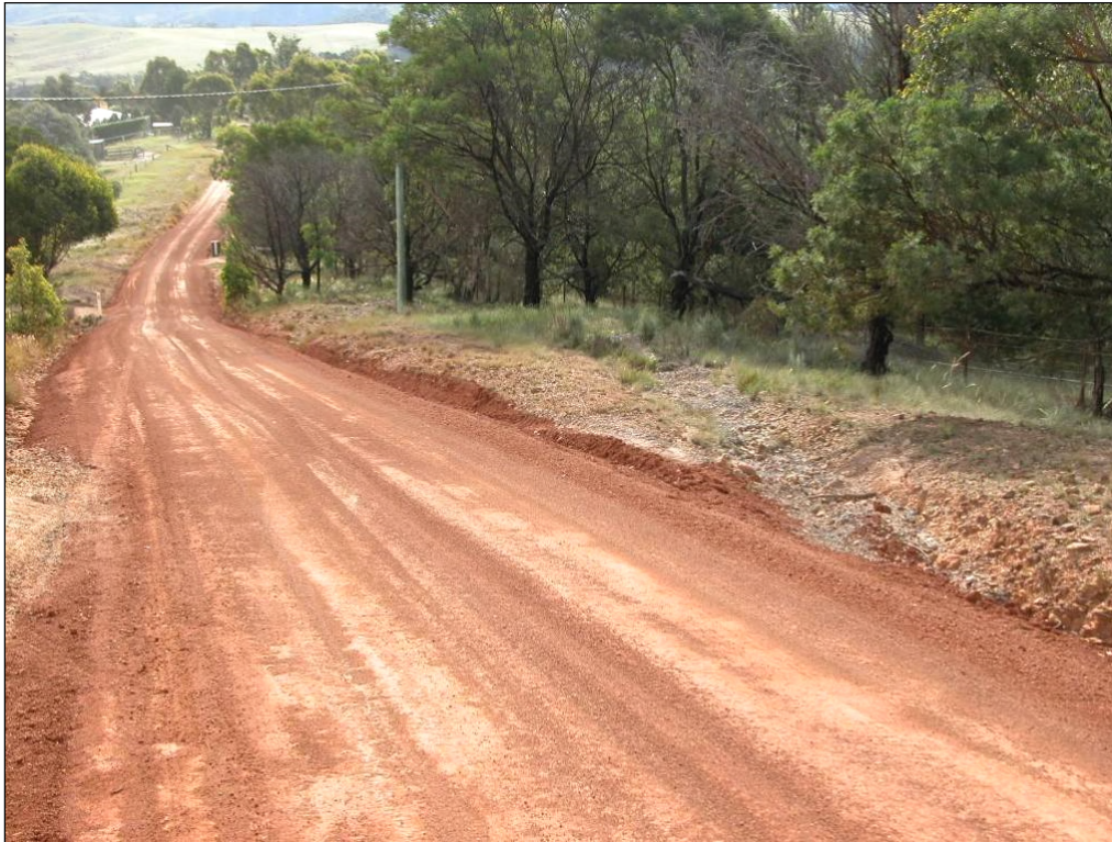
Figure 3-4 This ridge-line road required little cut and fill, and frequent turnout drains (two in the space of 30 m) divert stormwater to prevent erosion (NB: it is too steep for swales).
