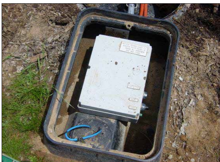
Figure 5.8 An electrical box that was flooded
