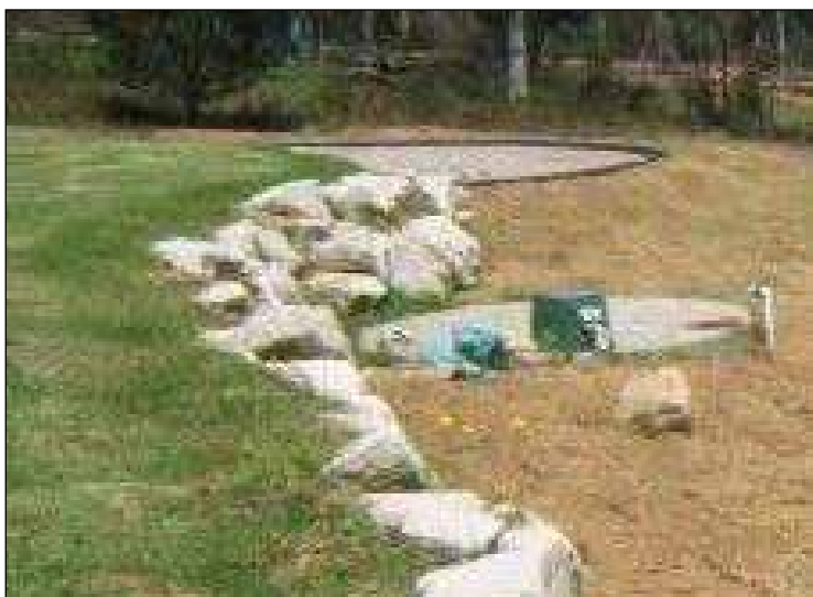
Figure 13.9 One of the new zones at the rear of the property established upslope of the aerated wastewater treatment system on imported soil
