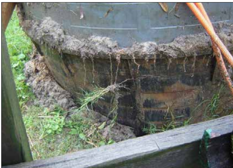
Figure 3.8 Tank that has lifted due to high water table
