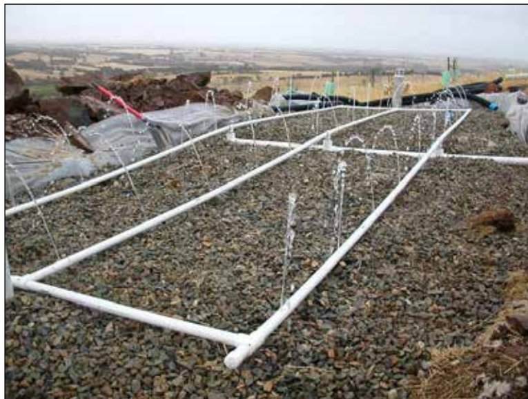
Figure 11.3 Pressure testing the distribution laterals for even distribution of effluent (Source: D Stafford)
