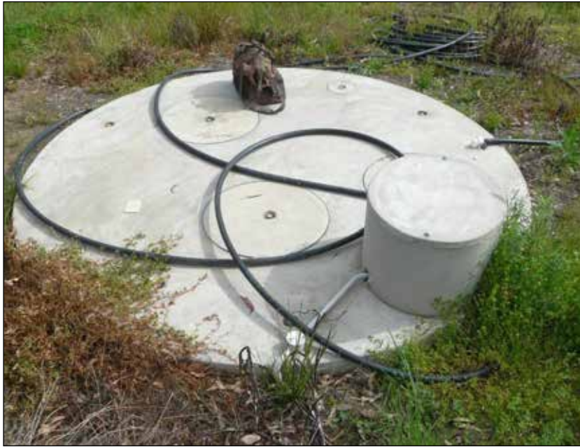
Figure 12.3 A surface irrigation system left coiled on top of treatment tank
