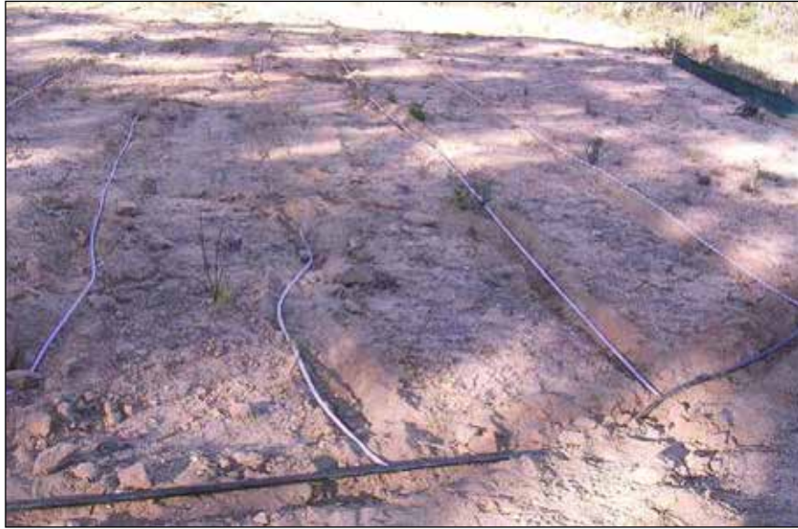
Figure 13.6 Poorly installed subsurface effluent irrigation system
