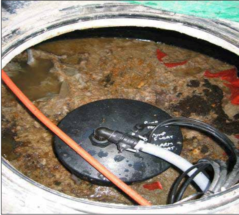
Figure 5.10 A flooded system due to pump failure
