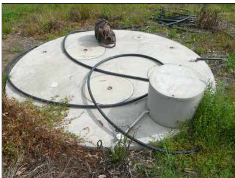
Figure 4.9 New AWTS with irrigation hose coiled on top, no sprinklers and potential for stormwater inundation
