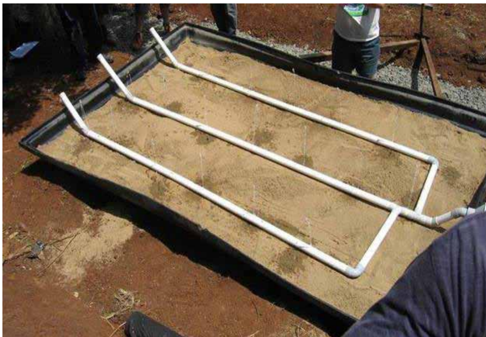
Figure 14.3 Siphon being tested delivering pressure dosed load to a sand filter (Whitehead & Associates)
