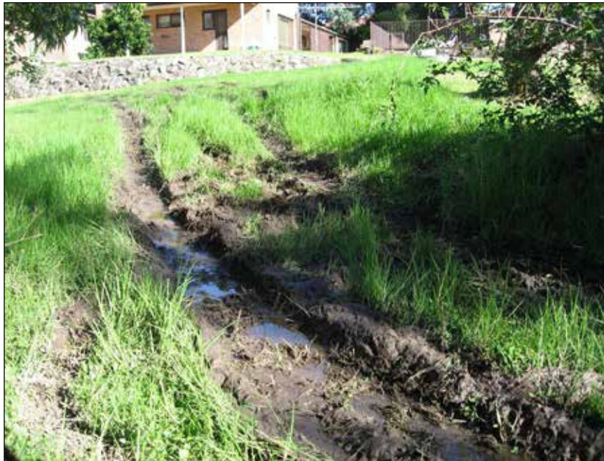
Figure 10.7 A failing trench due to vehicular activity
